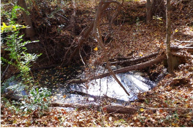
Photograph 5-7: Outlet pipe and resulting erosion downstream of earthen dam
