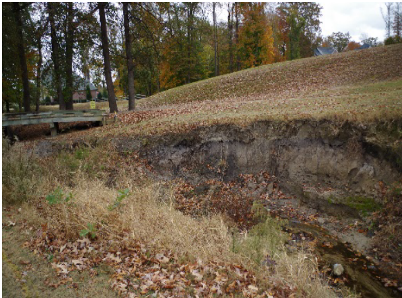
Photograph 5-2.: Bank Erosion on Right Bank Facing Downstream
