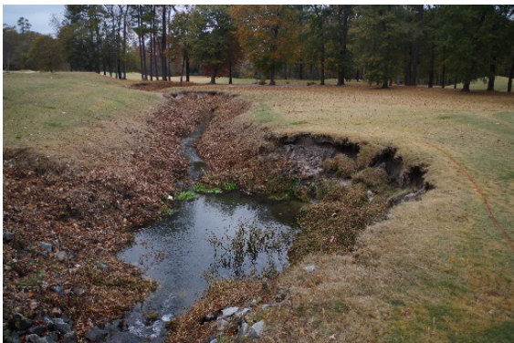
Photograph 5-1: Bank Erosion on Right Bank Facing Downstream
