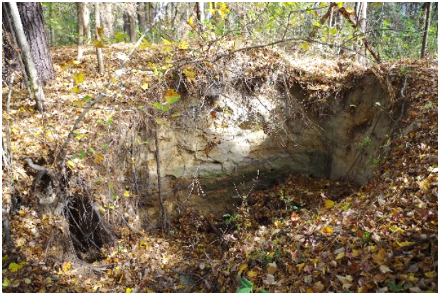
Photograph 5-6: Earthen Dam Failing
