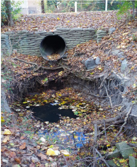
Photograph 5-8: Plunge pool formation at Beasley Dr. culvert
