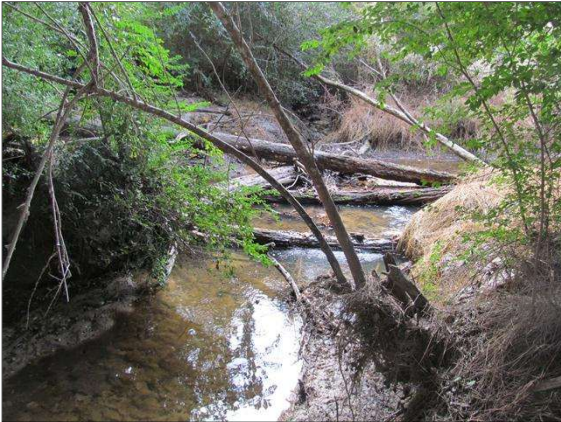
(PM)-VIEW LOOKING UPSTREAM AT DIVERSION DUE TO OBSTRUCTED WATERWAY IN SPAN 2.
