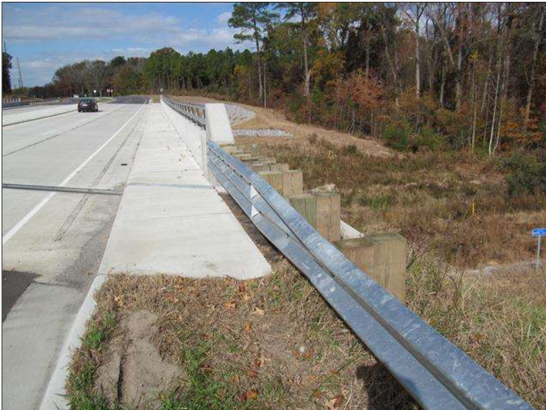
SE GUARDRAIL POST SPACINGS AT TRANSITION TO BRIDGE RAIL. (NE & NW TRANSITIONS SIMILAR, NO GUARDRAIL AT SW CORNER)
