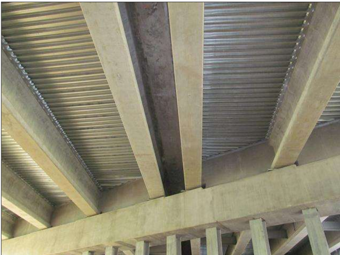
DECK UNDERSIDE IN SPAN 3 SHOWING GIRDER SPACING FOR G-5 & 6 AT CENTERLINE. THIS WAS A PHASED CONSTRUCTION.
