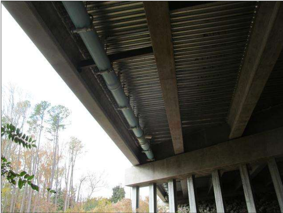
CLOSED DECK DRAINAGE SYSTEM ALONG BAY 1 IN SPAN 3. (SIMILAR IN ALL SPANS)
