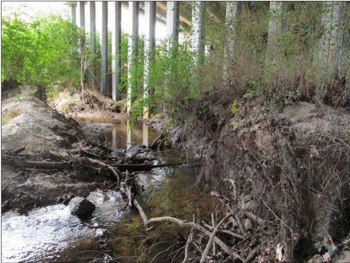
(PM)-VIEW SHOWING LOSS OF MATERIAL & LATERAL BANK MIGRATION AT SPAN 2 SIDE OF BENT 2, LOOKING UPSTREAM.
