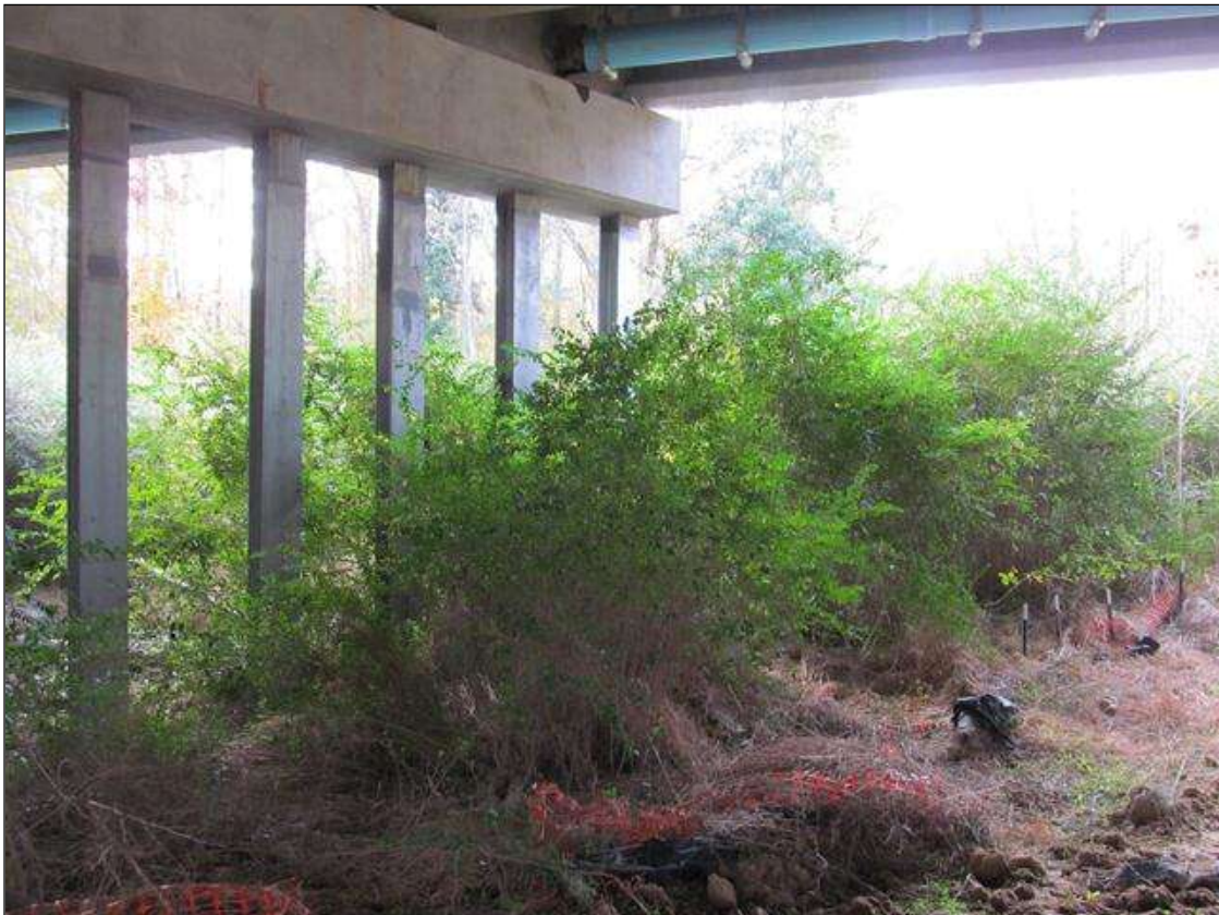
TREES AT SPAN 3 SIDE OF BENT 2
