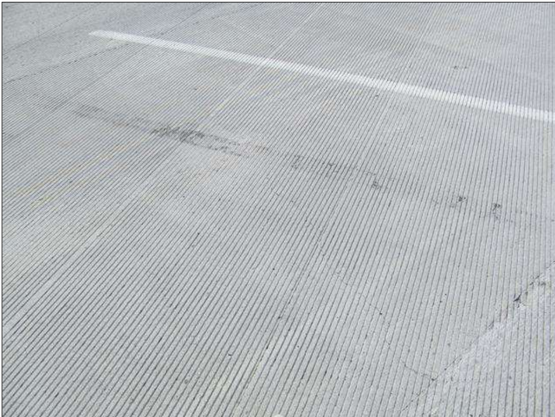
DECK OVER BT 1 IN NBL HAS DIAGONAL CRACKS TO 1/16". SIMILAR CRACKS IN BOTH LANES OVER ALL INTERIOR BENTS.
