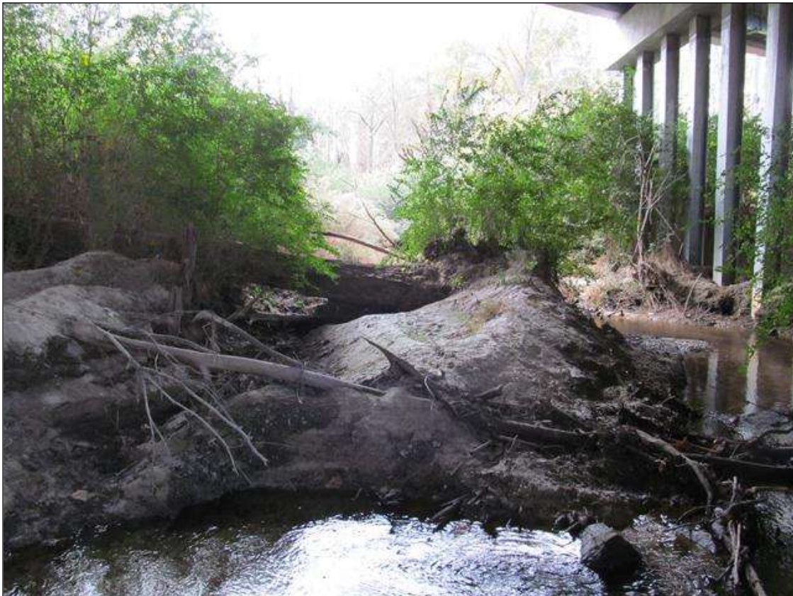
(PM)-CLOSE UP VIEW OF DRIFT/TREES & SILT BUILD UP IN CHANNEL OF SPAN 2.
