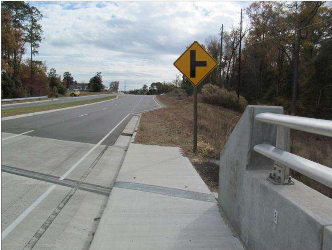
NO GUARDRAIL AT THE SW CORNER
