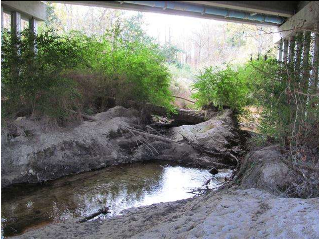
(PM)-LARGE TREES & DRIFT HAS CAUSED SILT BUILD UP AND DIVERSION OF FLOW AND LATERAL BANK MIGRATION (SCOUR) INTO SPAN 2 SIDE OF BENT 2.
