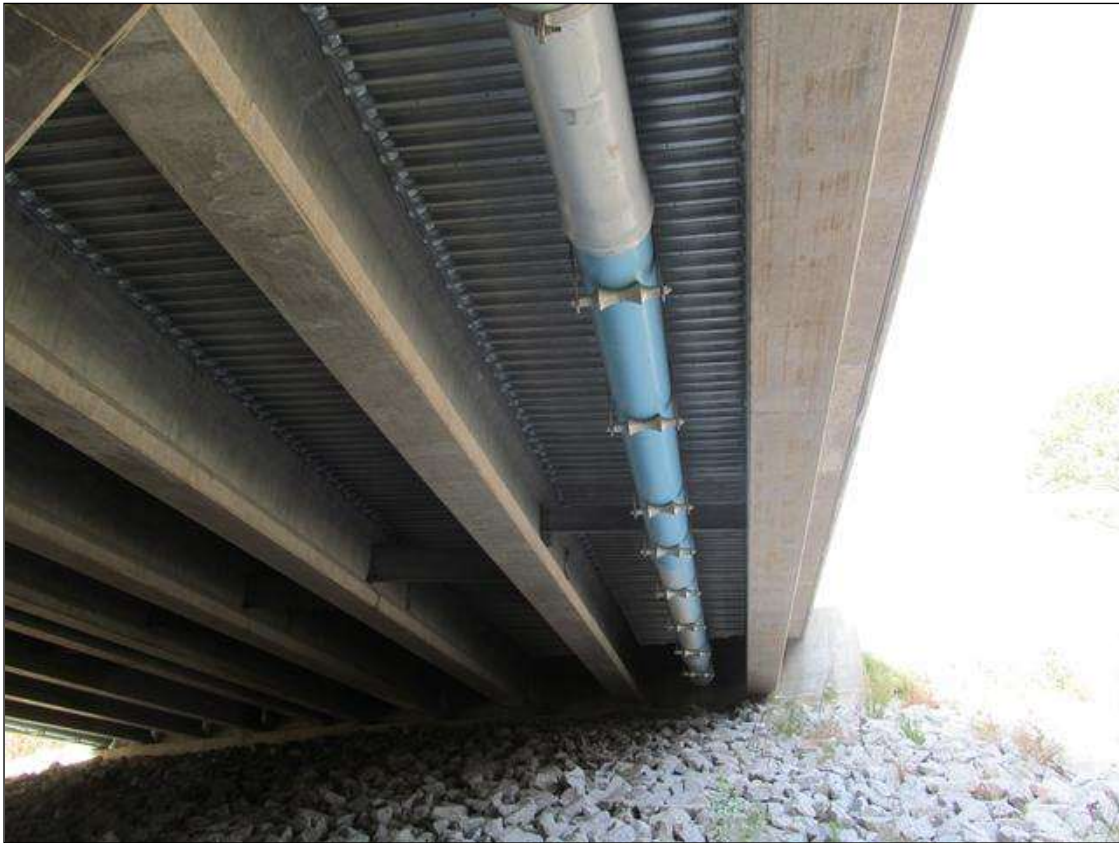
CLOSED DECK DRAINAGE SYSTEM ALONG BAY 9 IN SPAN 4. SIMILAR IN ALL SPANS.
