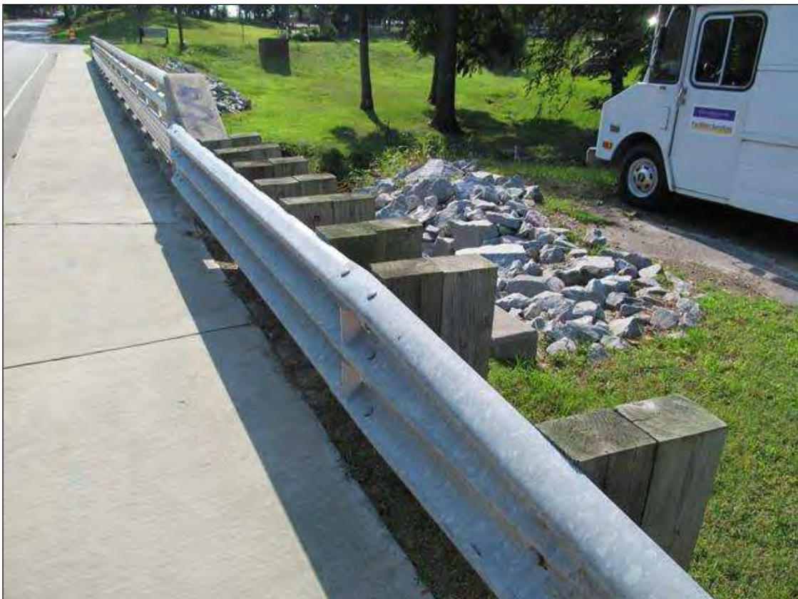
SW GUARDRAIL POST SPACINGS AT TRANSITION TO BRIDGE RAIL. (NE TRANSITION SIMILAR)
