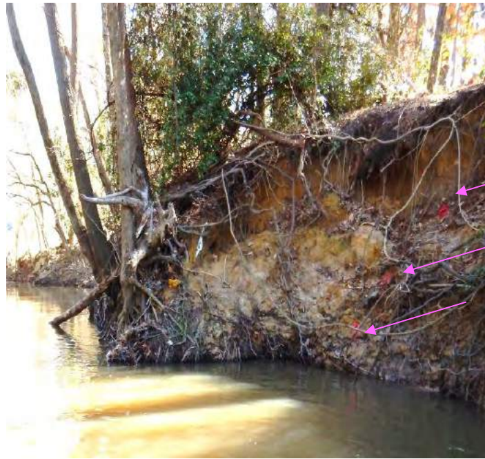
Picture 5-40: Extreme Bank Erosion
