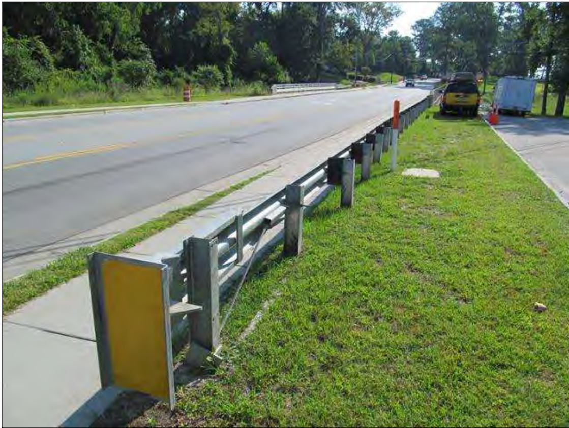
SW GUARDRAIL END TERMINAL. (NE END SIMILAR)
