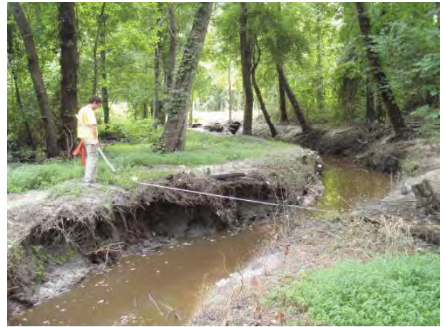
BEHI 1.1 Looking Downstream
