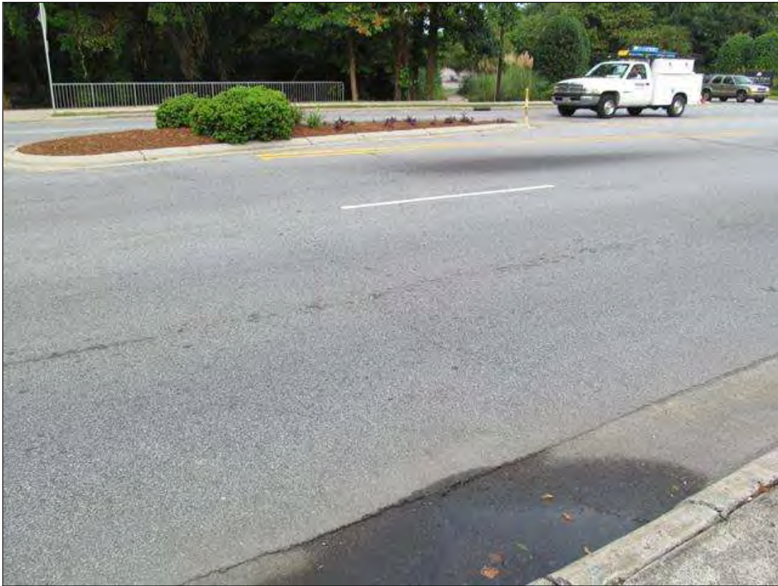
NORTH BOUND LANES @ THE SOUTH APPROACH CRACKED WITH SETTLEMENT. SIMILAR IN ALL LANES @ BOTH APPROACHES.
