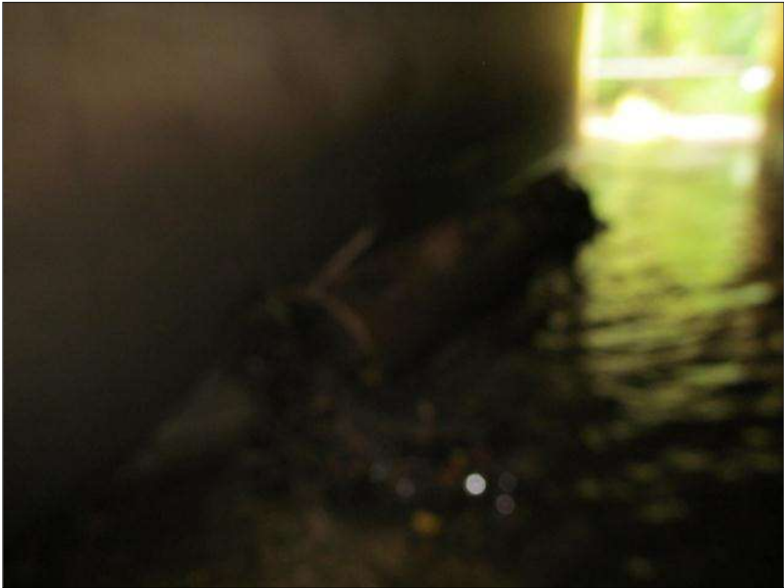
PIPE & DEBRIS IN BARREL 3
