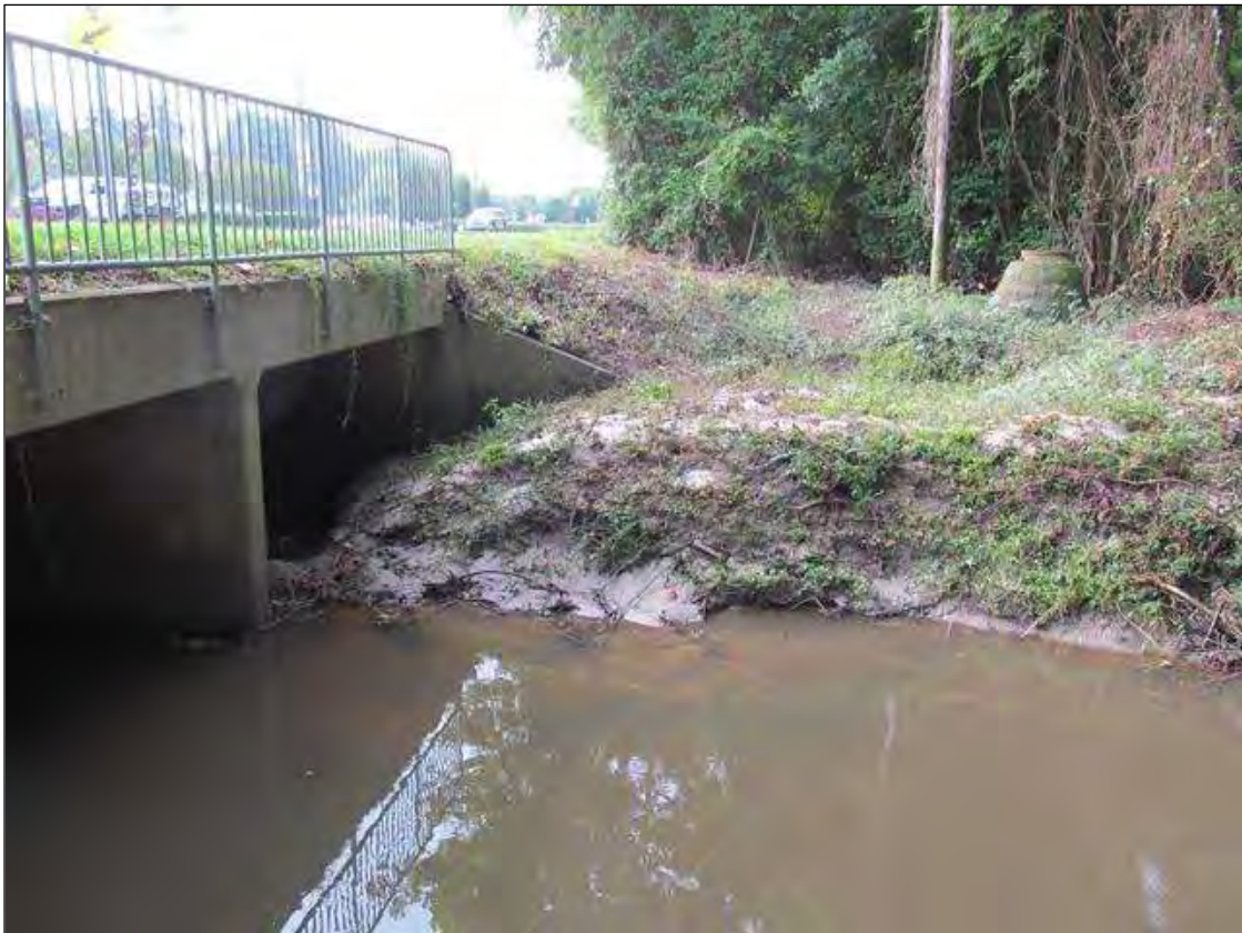
SILT @ THE WEST END OF BARREL 1.
