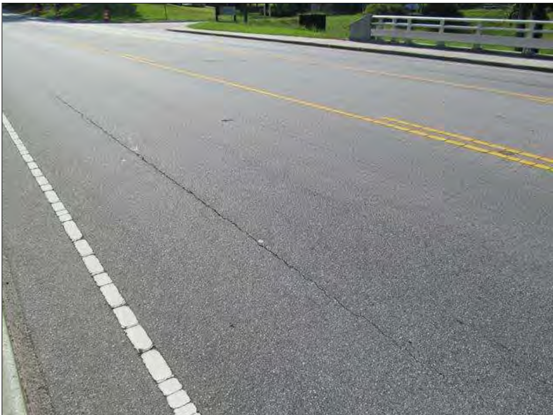
SIMILAR LONGITUDINAL CRACKS IN LT LANE OF SPAN 2. SIMLAR AT RT LANE & C/L OF SPAN 1.
