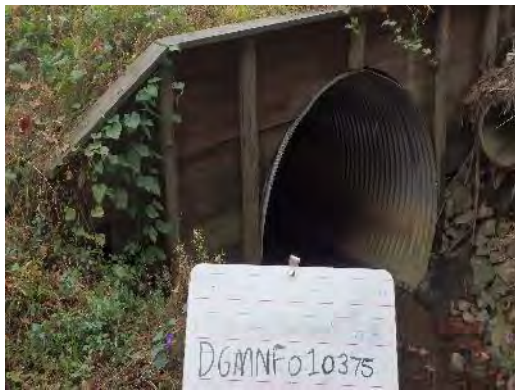
Picture H- 15. North Fork to Greens Mill Run: Allen Road Upstream Face
