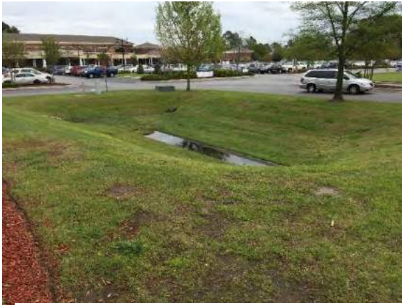
Picture 5-35: Arlington Crossing Shopping Center Wet Detention Basin Retrofit (North)
