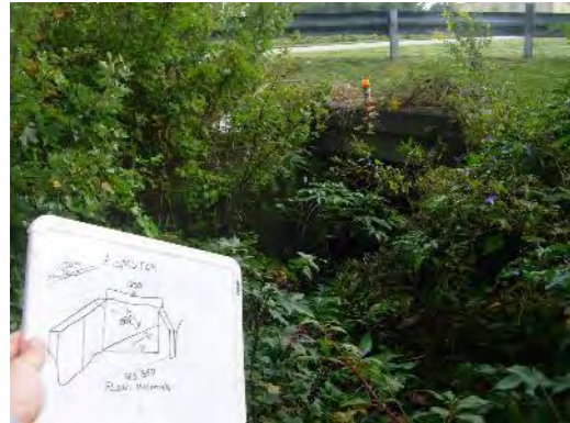
Picture H- 22. Unnamed Tributary to Greens Mill Run: Greenville Boulevard Upstream Face
