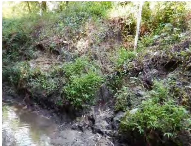
Picture 5-7: Left Stream Bank Erosion
