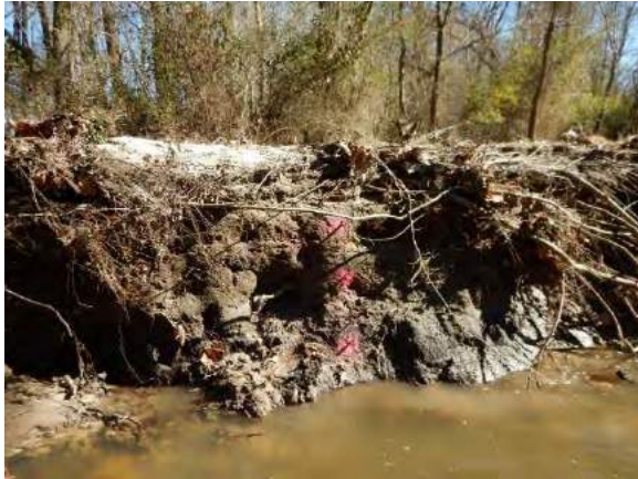
Picture 5-3: Stream Bank Erosion and Pins at Installation
