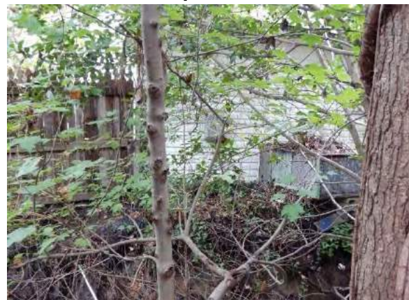
Picture 5-13: Threatened Structures Near Top of Bank
