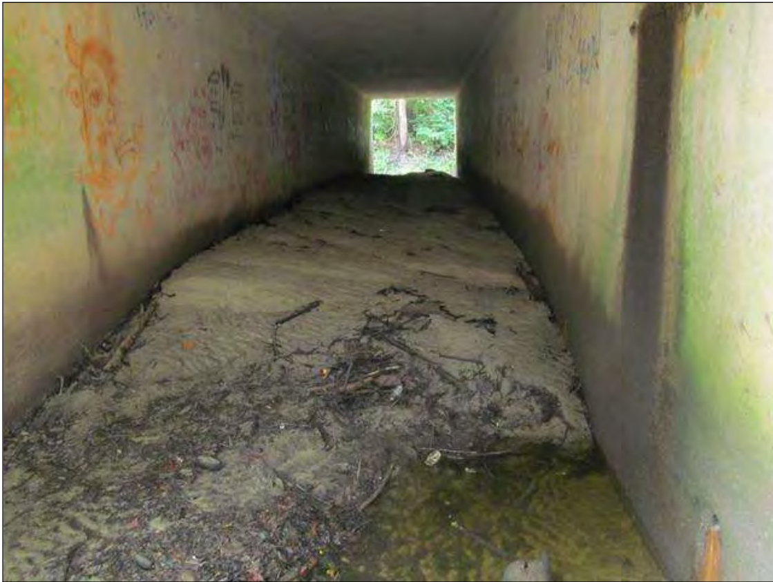
SILT IN BARREL 1.
