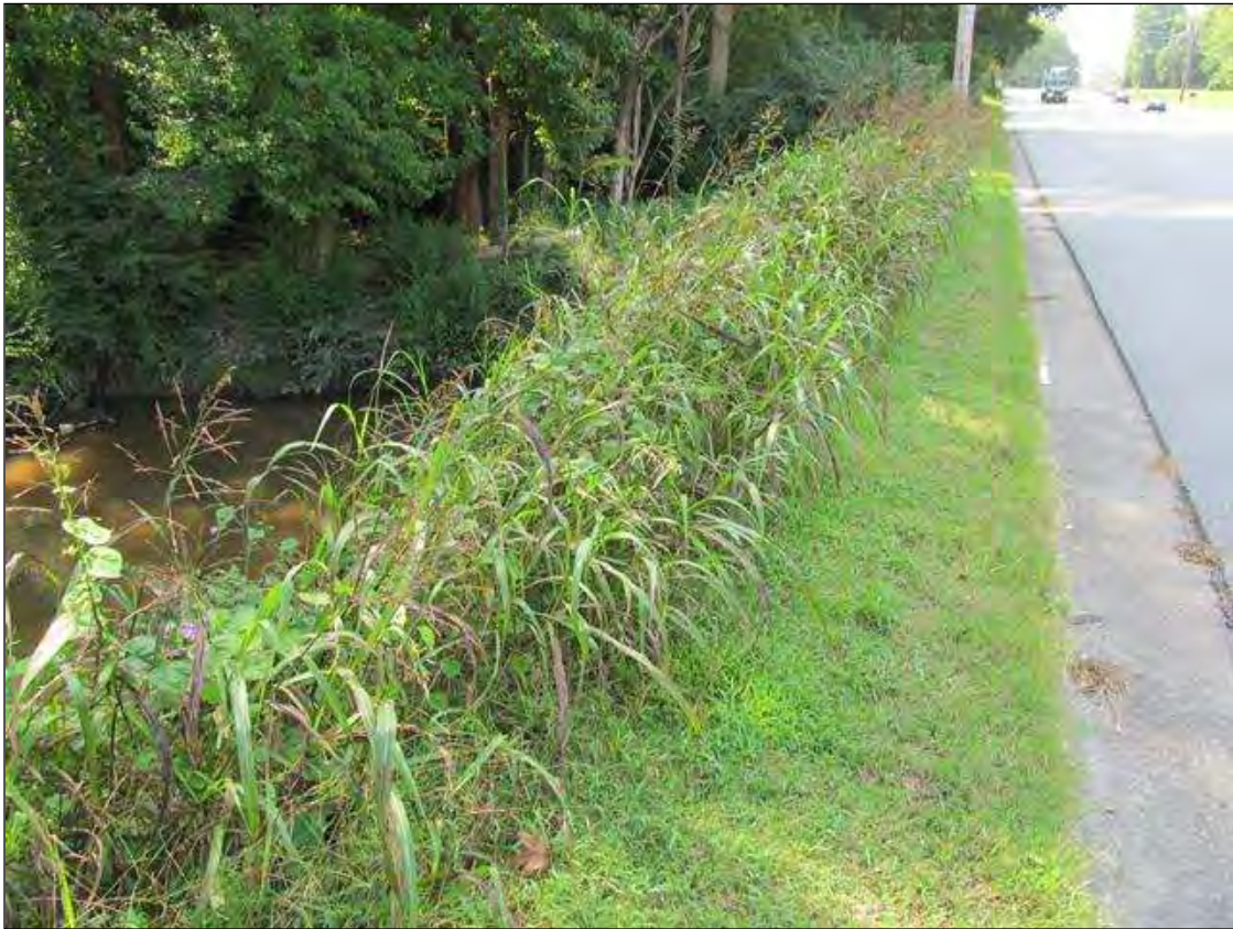
HEAVY VEGETATION ALONG THE EAST HEADWALL.
