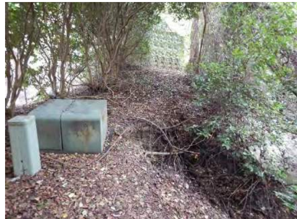
Picture 5-12: Electric Transformers at Top of Bank
