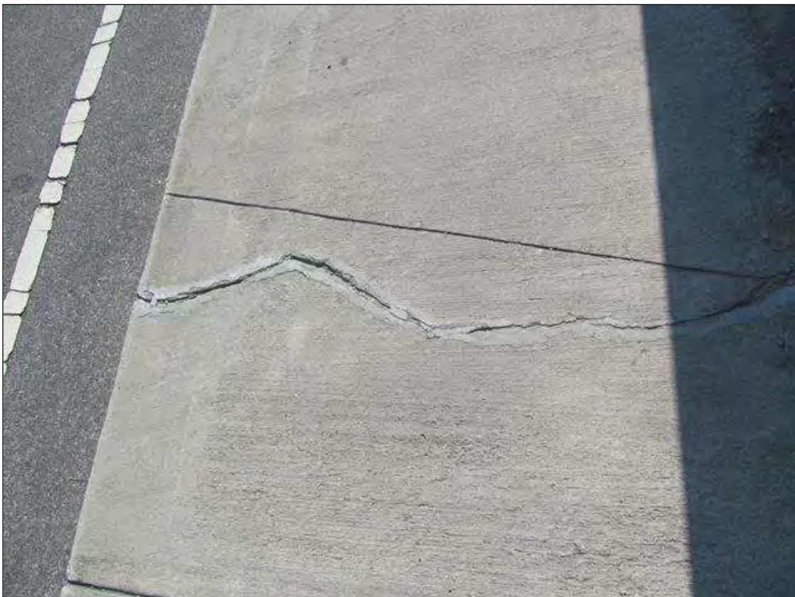
TRANSVERSE CRACK VISIBLE THRU FAILED PATCH MATERIAL ALONG RT WALKWAY. SIMILAR AT LT SIDE.
