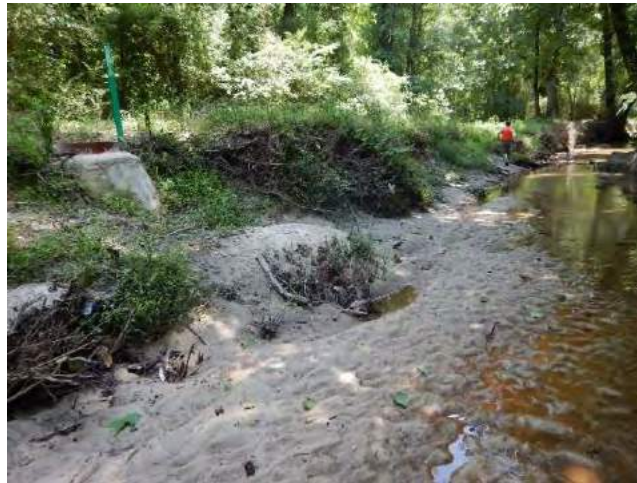
Picture 5-1: Exposed Manhole and Stream Bank Erosion
