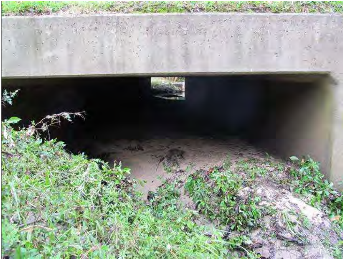
SILT IN BARREL 1. SIMILAR IN BARREL 3 @ THE EAST END.
