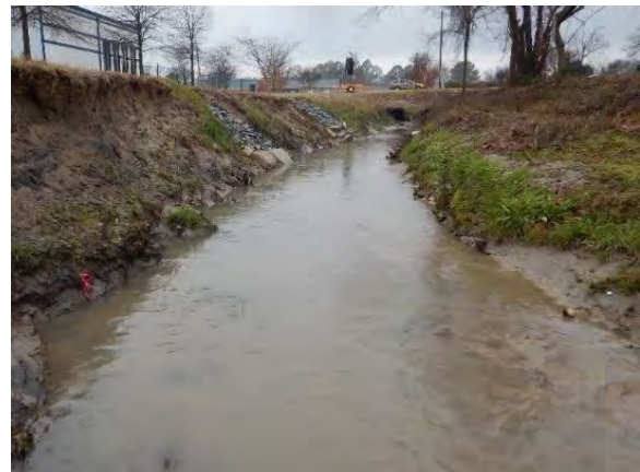
Picture 5-10: Stable Left Bank and Eroded Right Bank
