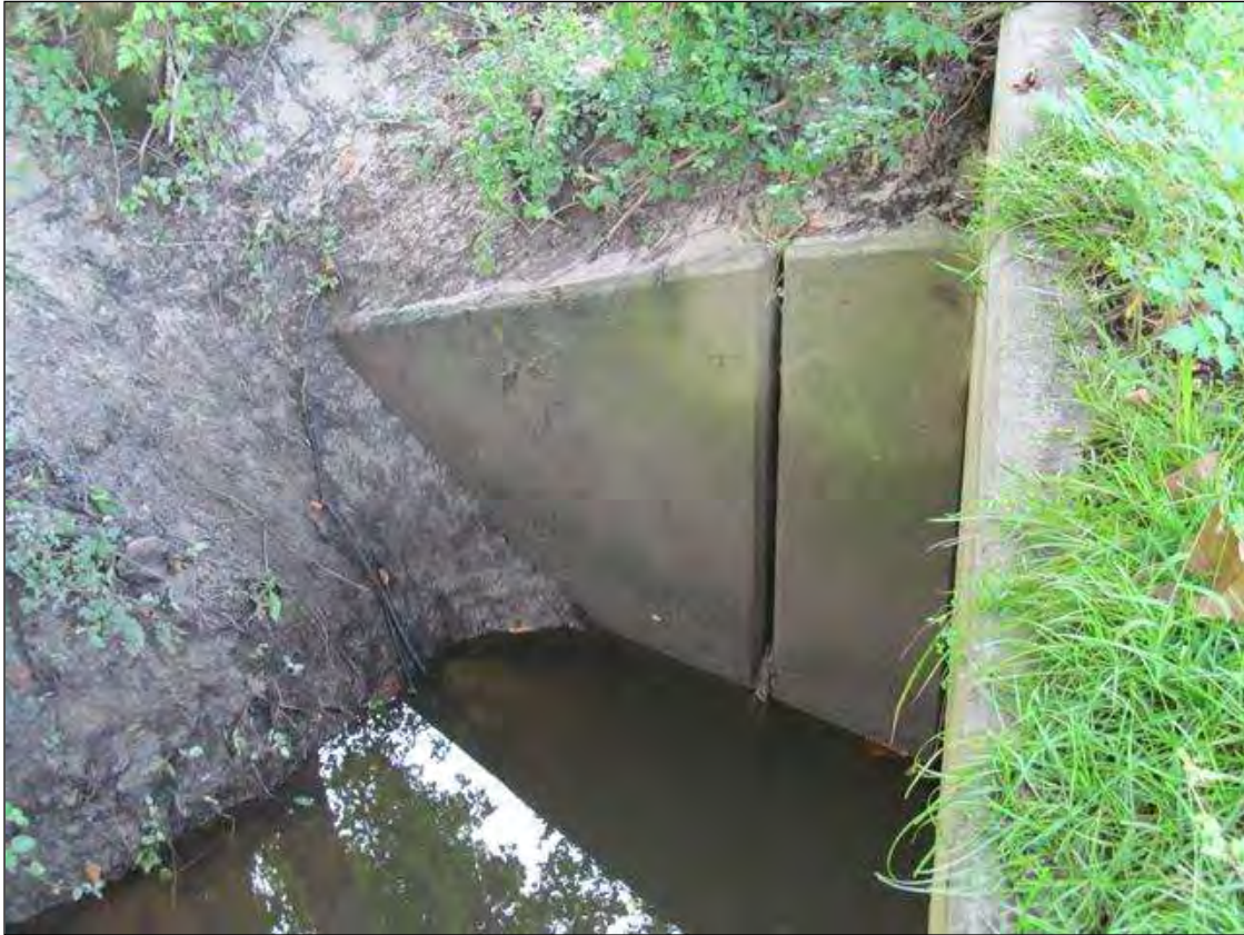
SE RETAINING WALL IS MISSING JOINT MATERIAL BETWEEN SECTIONS ALLOWING FILL LEAKAGE. SIMILAR AT ALL CORNERS.
