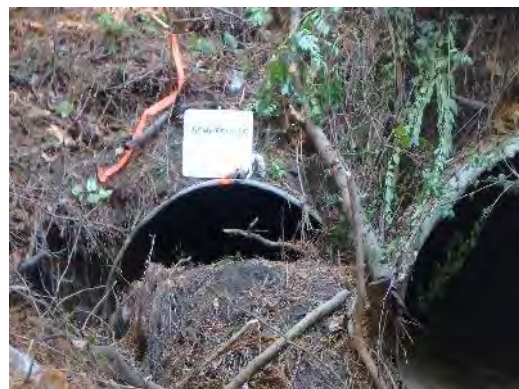
Picture H- 18. North Fork to Greens Mill Run: Ellsworth Drive Downstream Face
