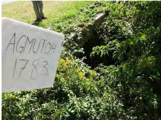
Picture H- 21. Unnamed Tributary to Greens Mill Run: Greenville Boulevard Upstream Face
