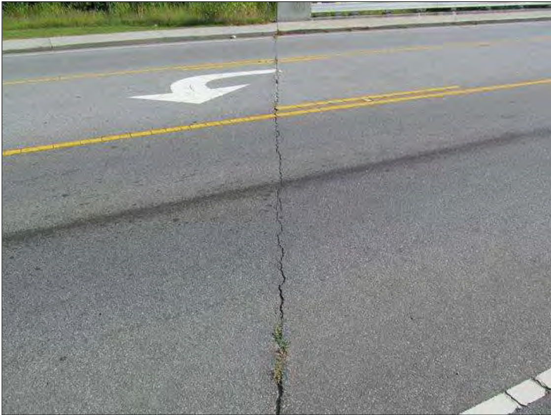
SIMILAR TRANSVERSE CRACKS IN WEARING SURFACE OVER SUPPORTS.
